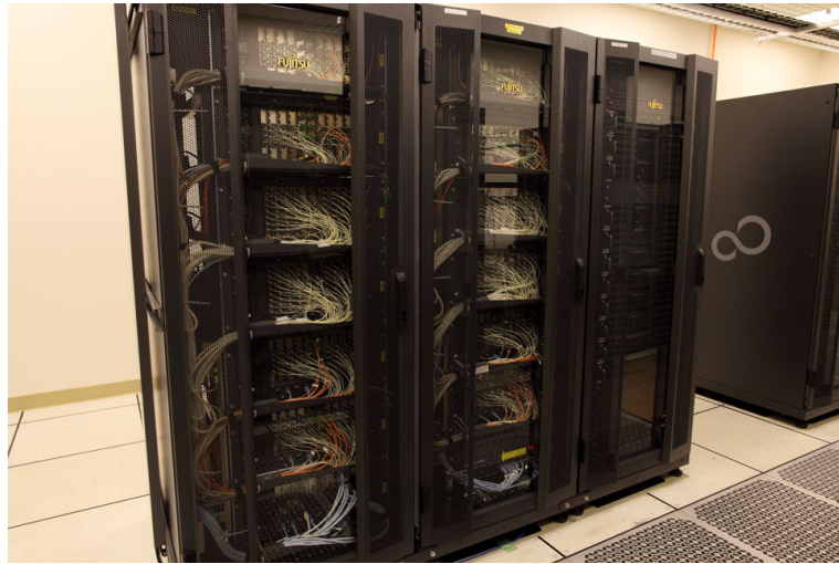
Figure 4.6: A quadrant of the ACA Correlator. The left and middle racks compose a quadrant, which processes a baseband pair from sixteen antennas. The right rack is one of four computing racks, which have correlator control, post processing computers, network instruments and so on.
